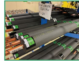
Insulated risers tested to 300 psi
