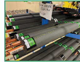
Insulated risers tested to 300 psi
